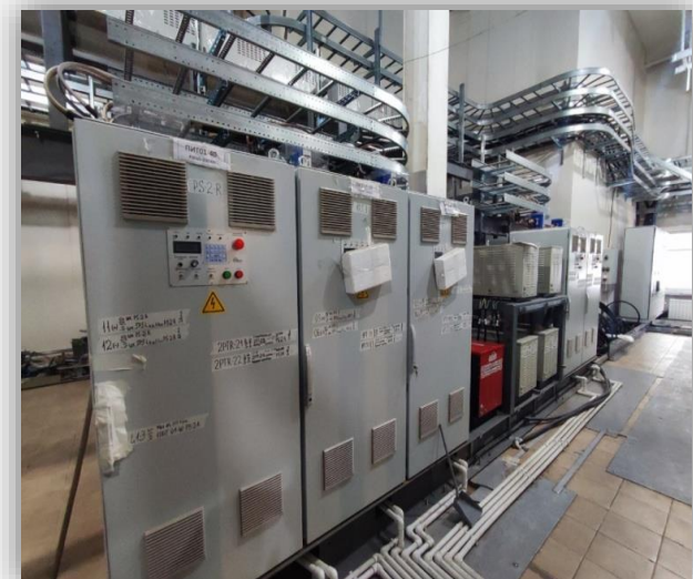
Main power supply units
