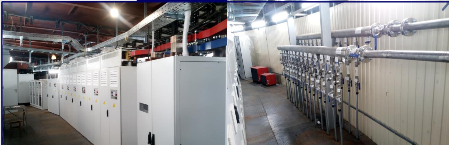
Booster PS system placed in the “cellar” under the Bldg No 1.
