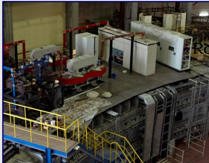
Booster PS placed on the top of the Synchrotron yoke
