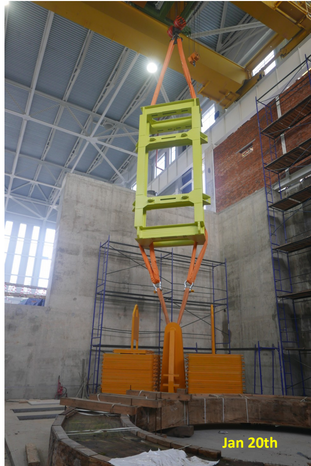
MPD Hall crane weight test
