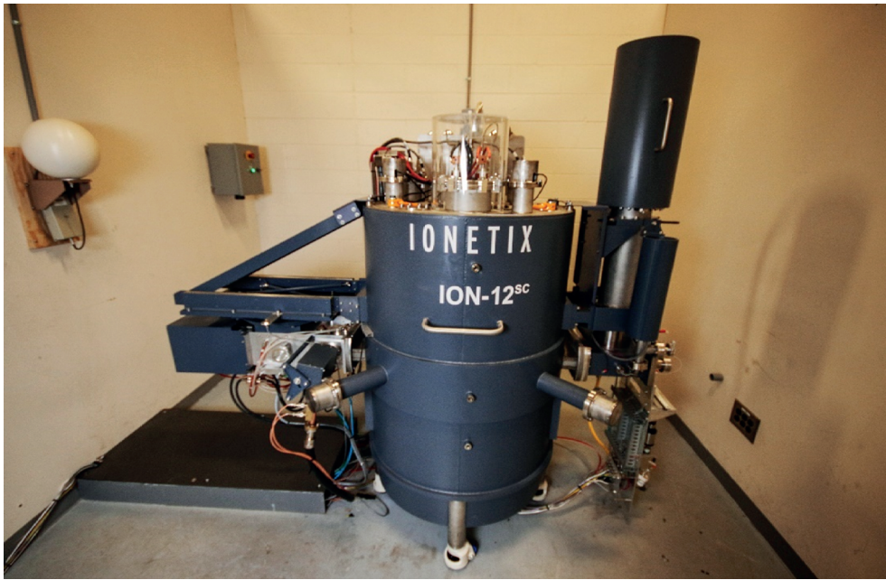
Fig. 1. Cyclotron installation with the equipment around shown.
