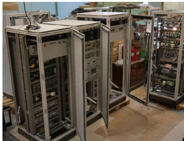
Blocks of electronics of the DC-280 control system
