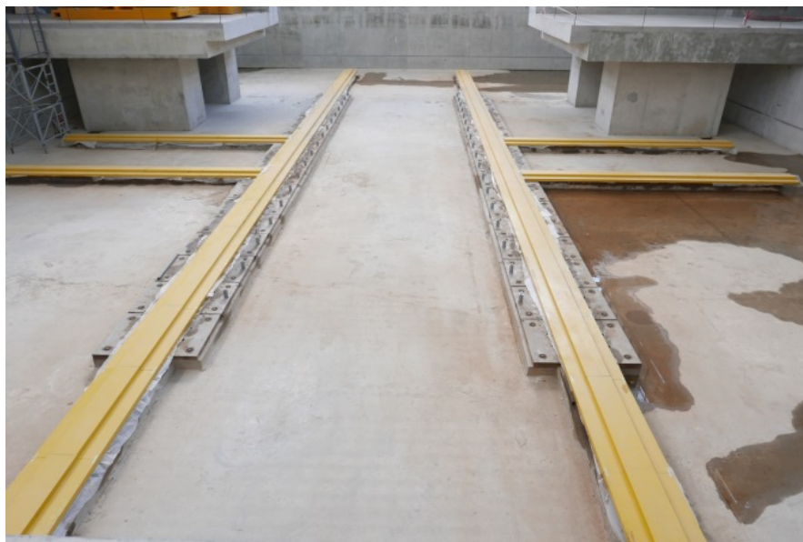
Fig. 2.2.1.17. Rail tracks in the pit of the MPD pavilion. Working surfaces are closed by casings.
