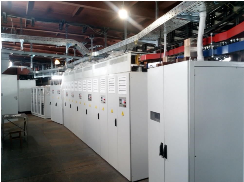
Fig.2.1.3.19. The Booster power supply units.
