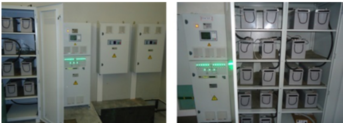
Puc. 2.3.7.3. Equipment for the reconstruction of the operational current system.
