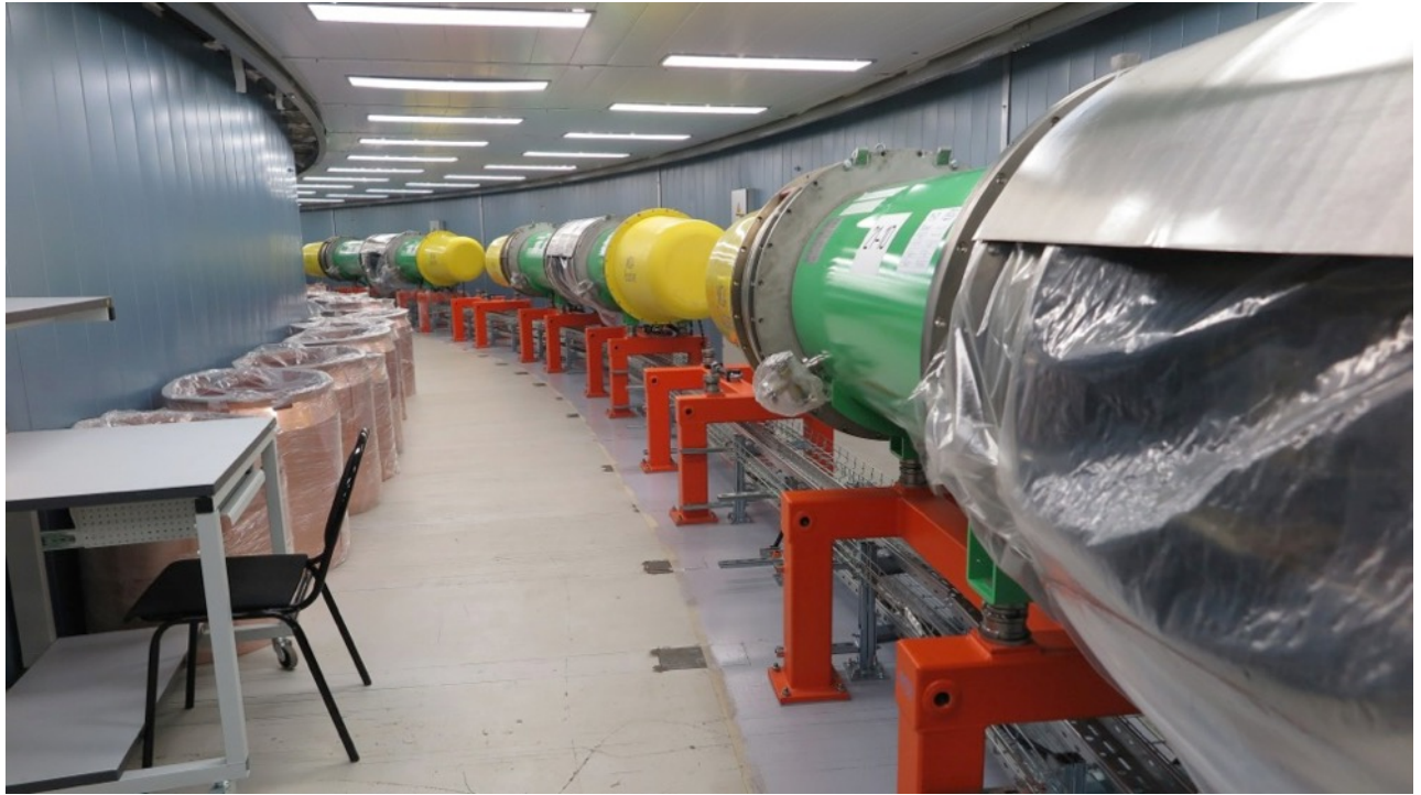
Puc. 2.1.3.4. Sections of the dipole magnets inside the tunnel.
