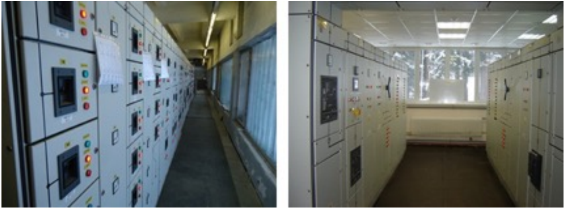
Puc. 2.3.7.4. Reconstructed switchgear of buildings No. 205 (left) and No. 217 (right).
