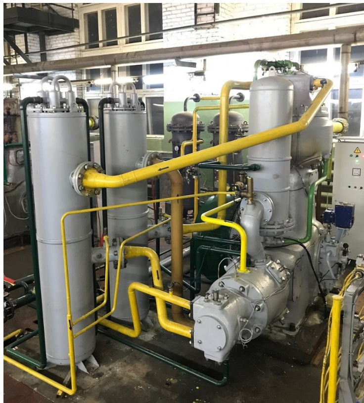
Fig. 2.3.6.2. Piston compressor “305NP-20/31”
