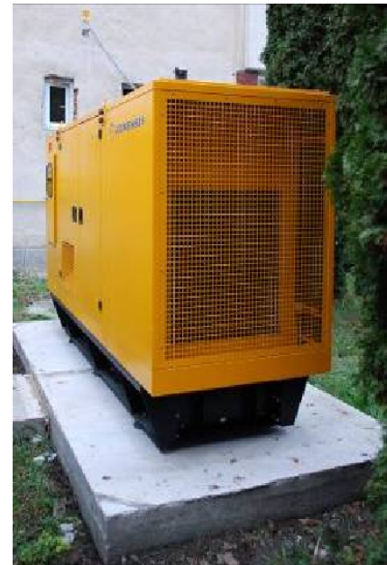
Power generator 275 kW
