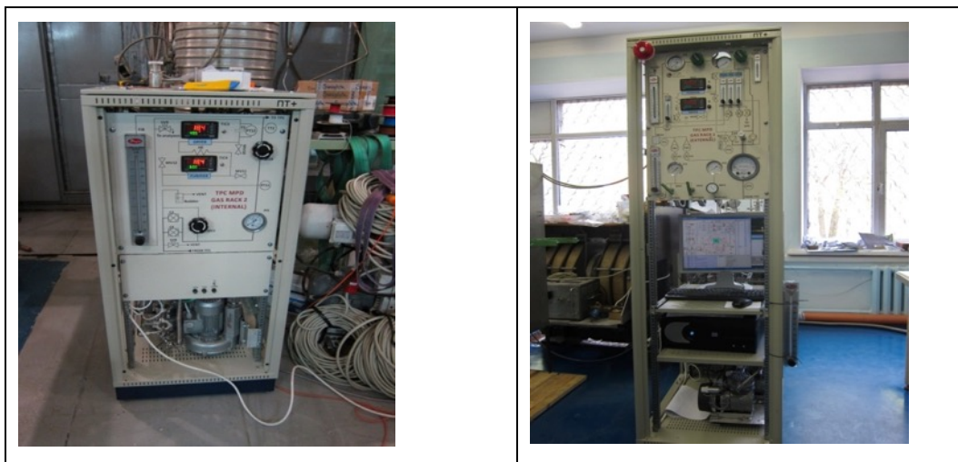
Fig. 3.3.2. Assembled rack 1 and rack 2 for gas system
