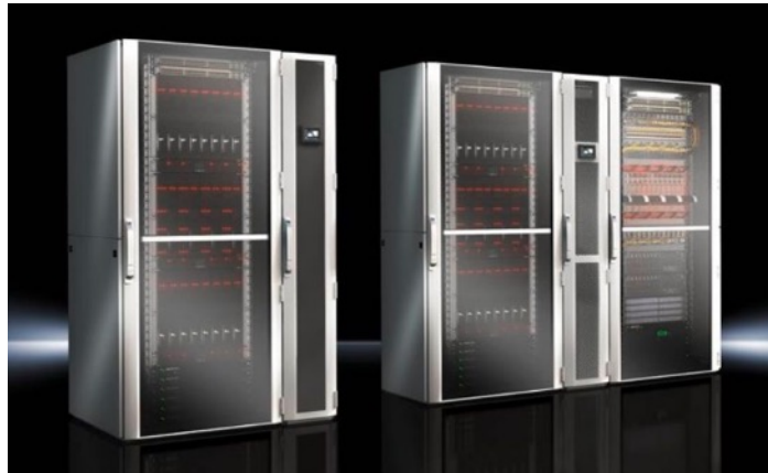
Fig. 3.11.2. RACK - the Main Module of the Mechanical Structure, AUXILIARY RACK - COOLING UNIT
