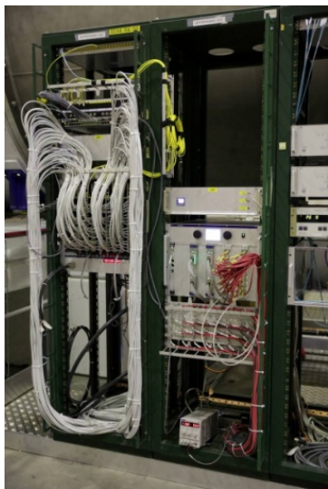
HV and LV power suppliers
