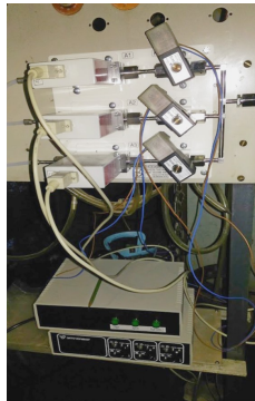
Figure 17: Electronic gas supply system of RPC.
