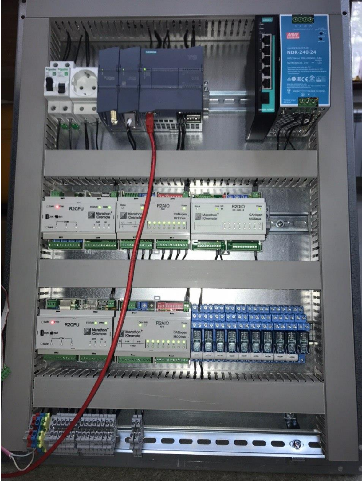
Gas station control
