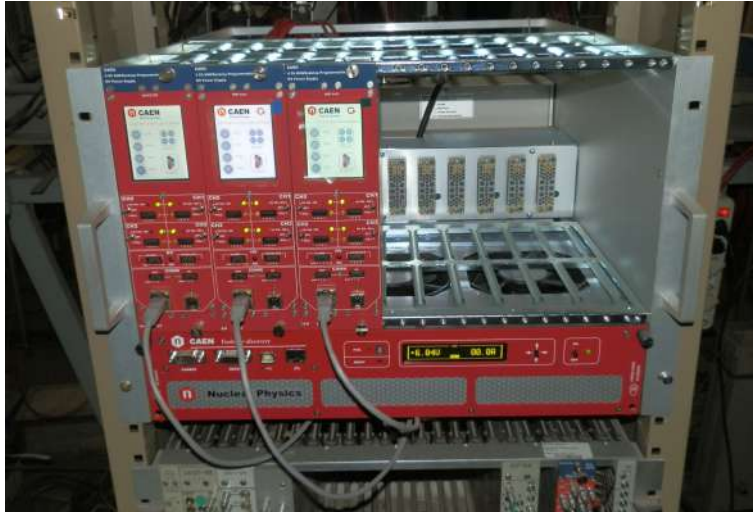
Figure 21: NIM crate with CAEN high voltage power supply for proportional chambers.
