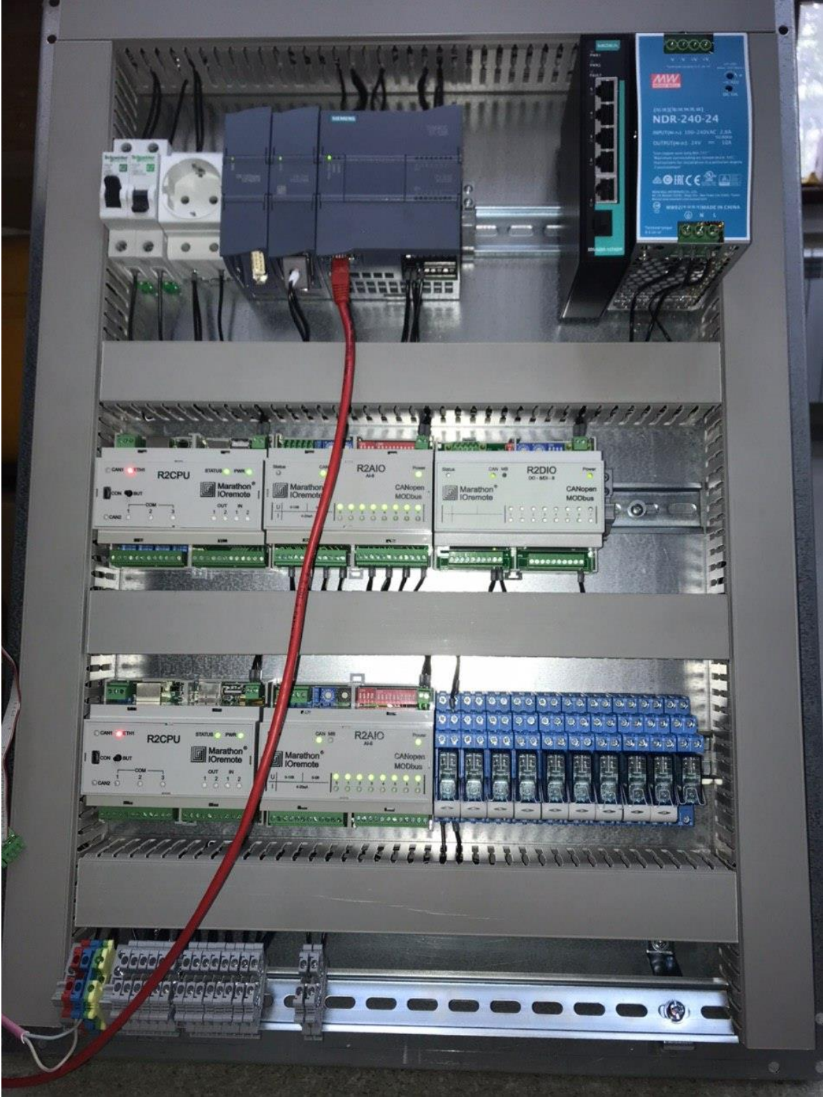
Gas station control
