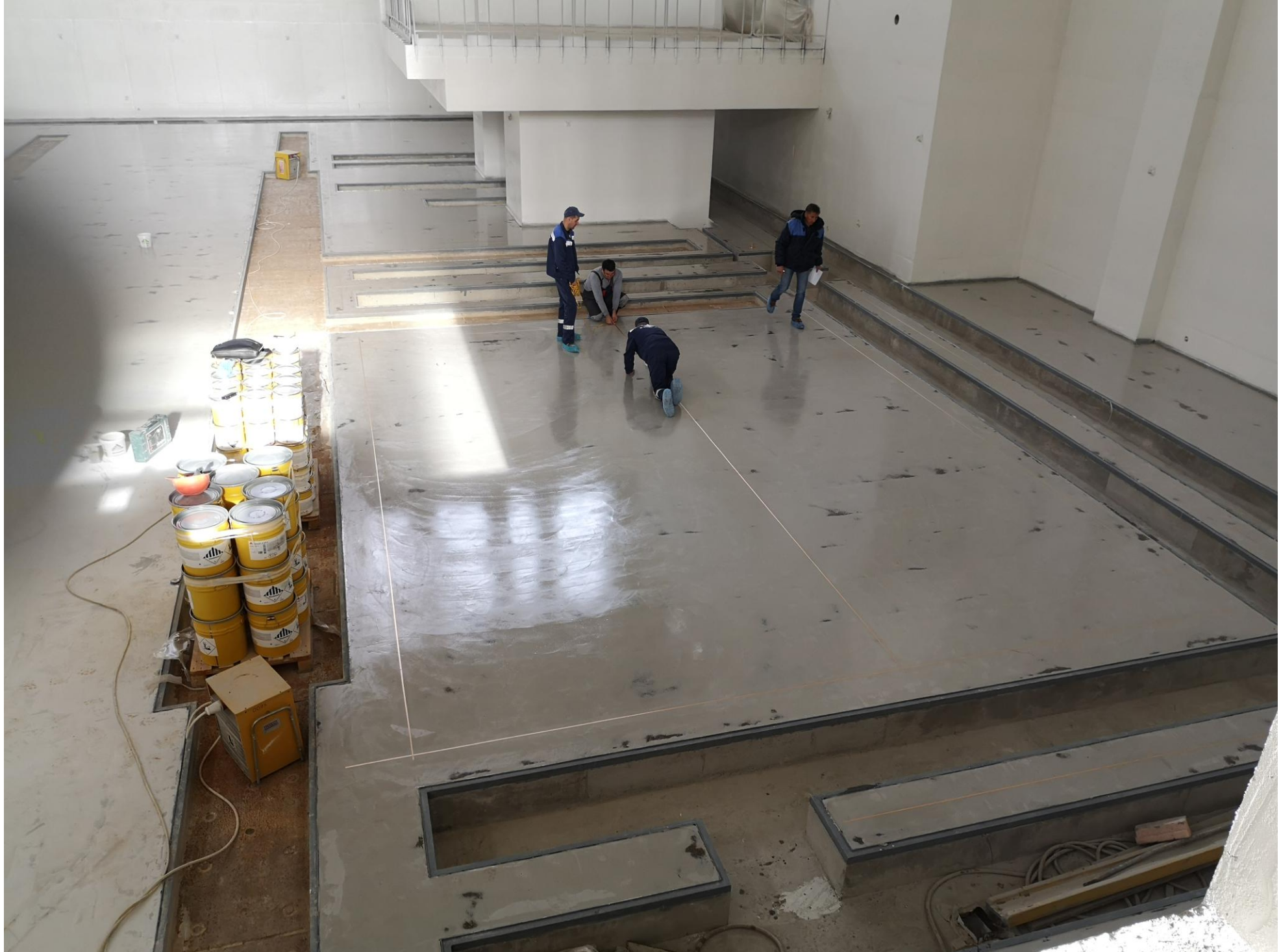
Self-leveling floors have been poured. Anti-static tape has been stuck into the floor over its entire surface: 20.10.2021
