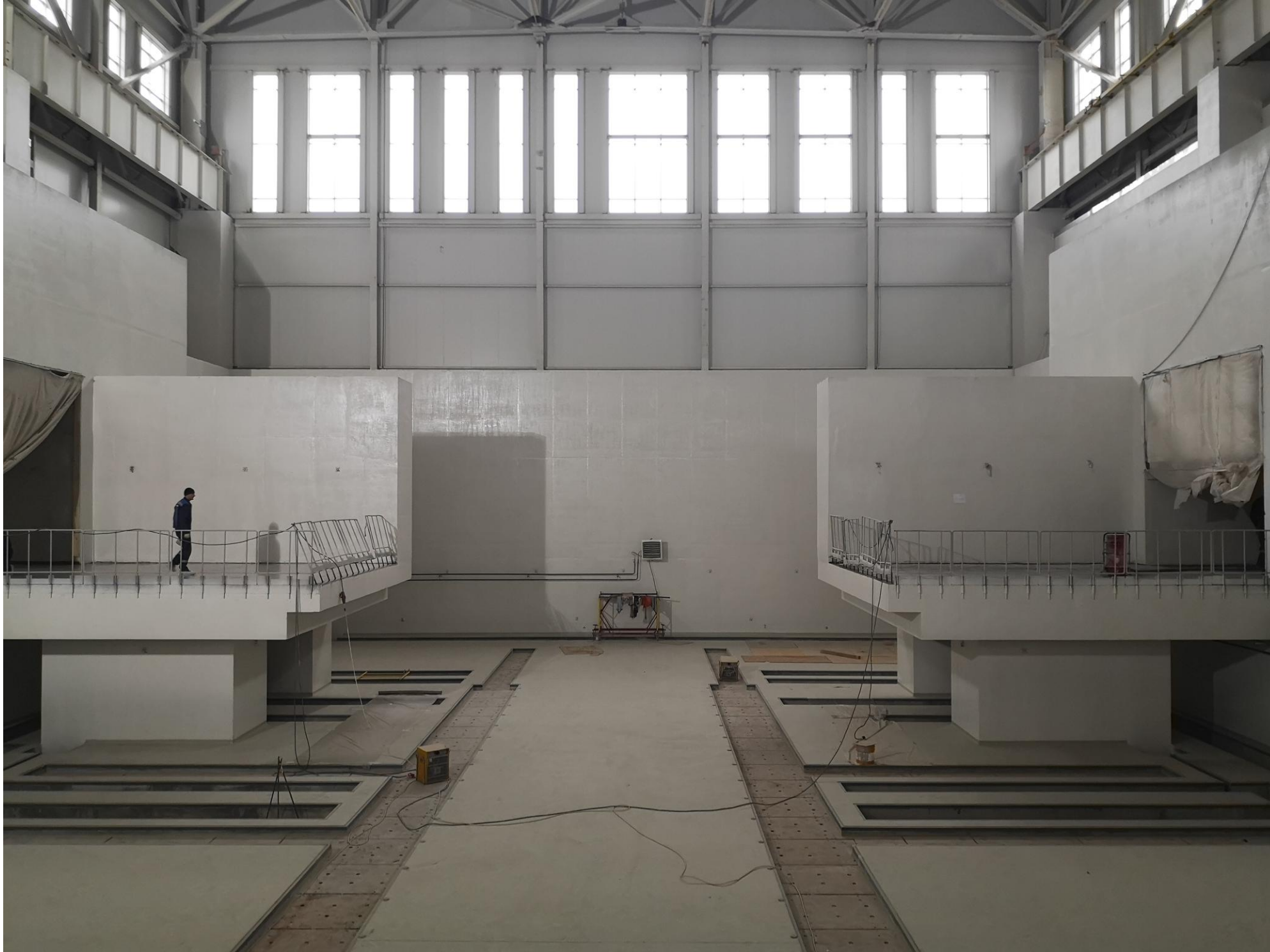
Work on the technological gutters in the concrete floor has been completed: 08.07.2021
