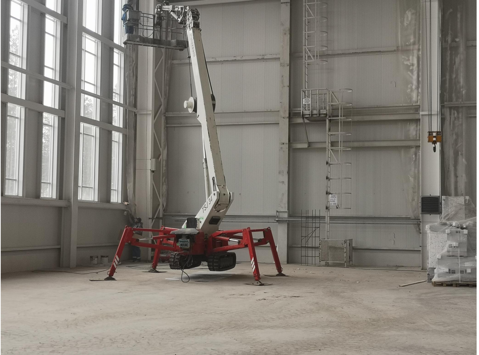
The interior painting of the walls of the hall is being completed.
