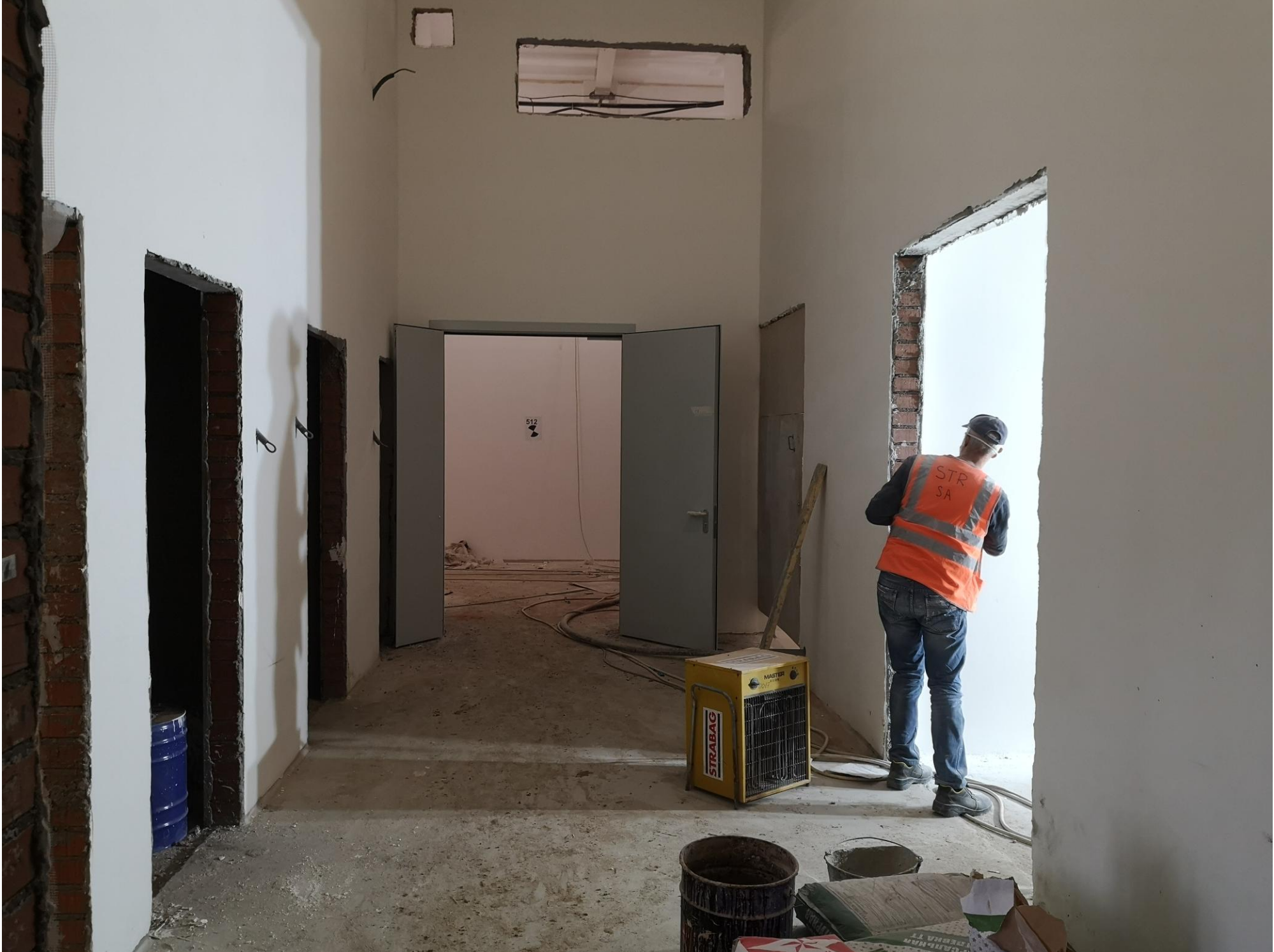
Interior decoration of the control room: 11.19.2021
