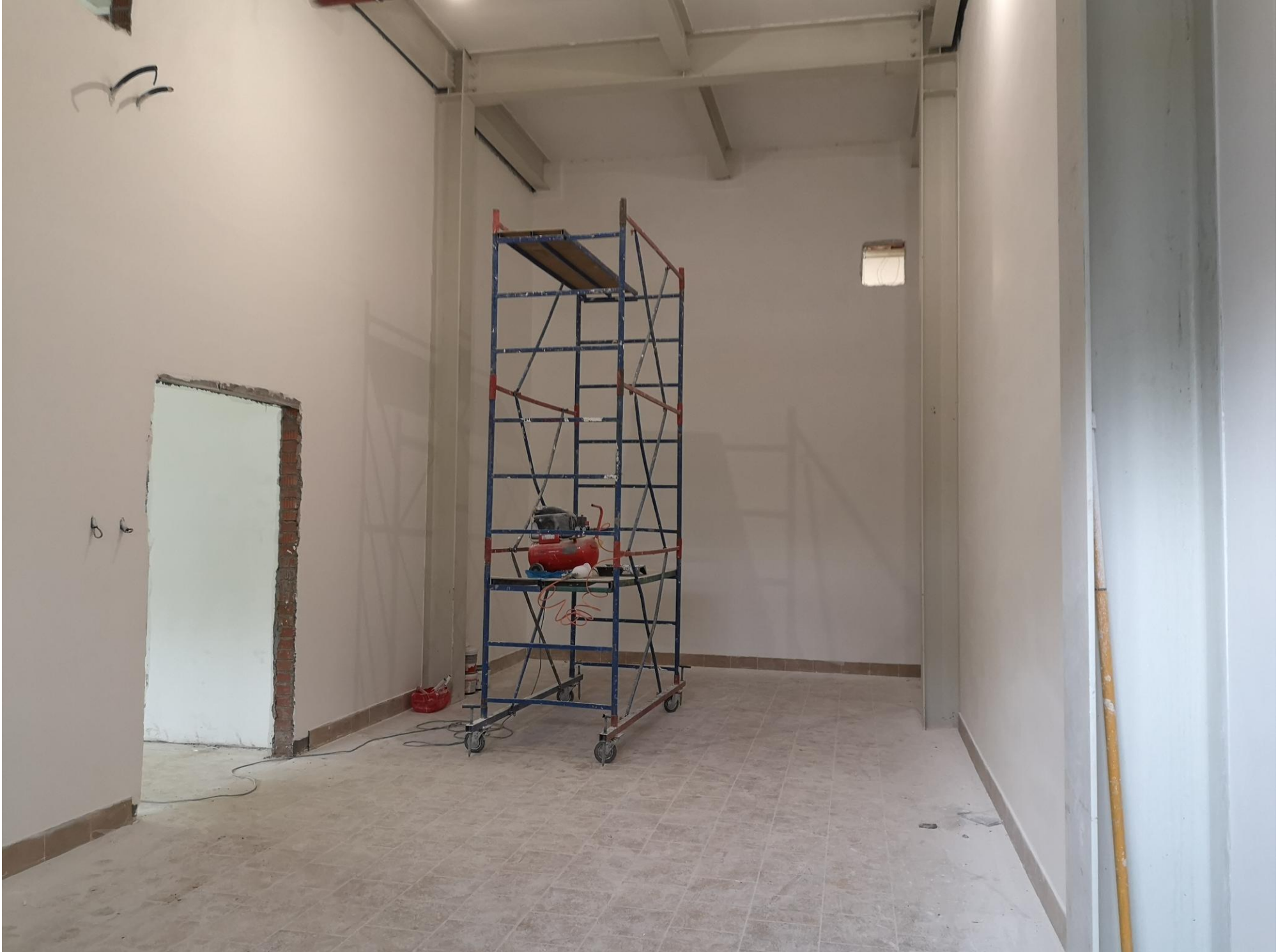
The interior decoration in the main control room is almost complete.
