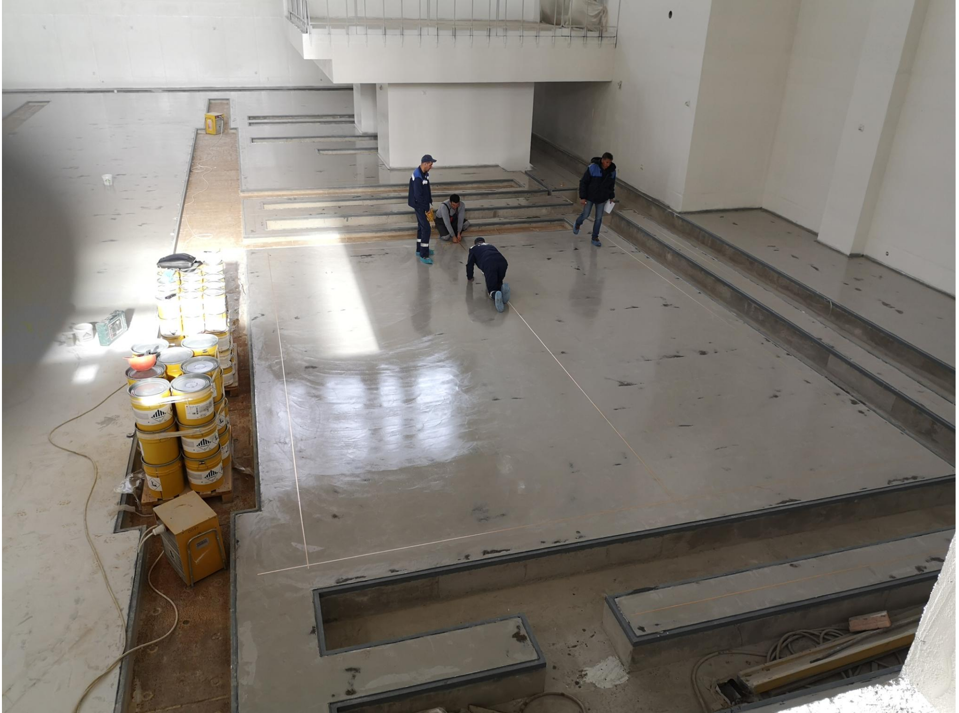
Self-leveling floors have been poured. Anti-static tape has been stuck into the floor over its entire surface: 10/20/2021
