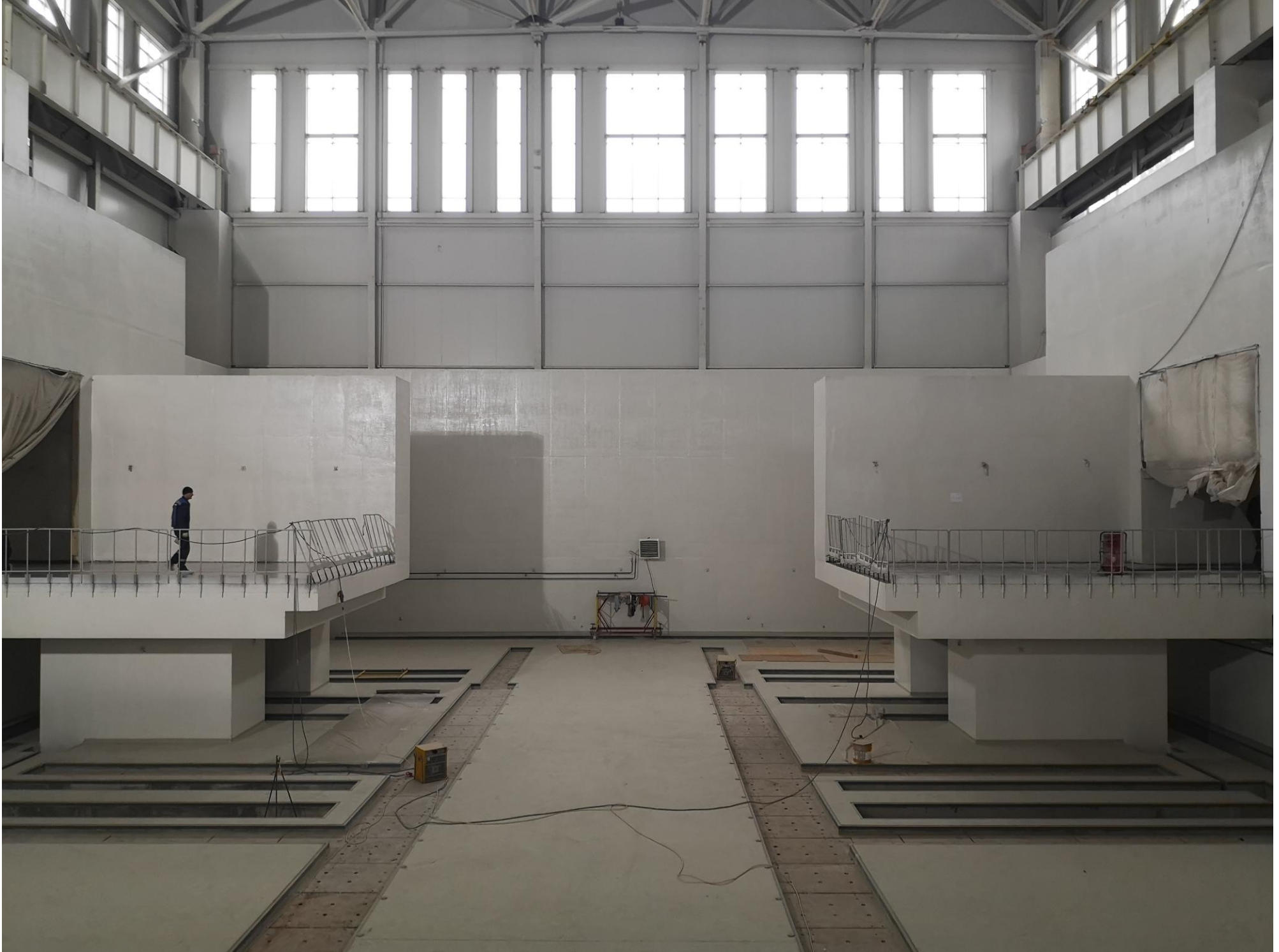
Work on the technological gutters in the concrete floor has been completed: 07/08/2021
