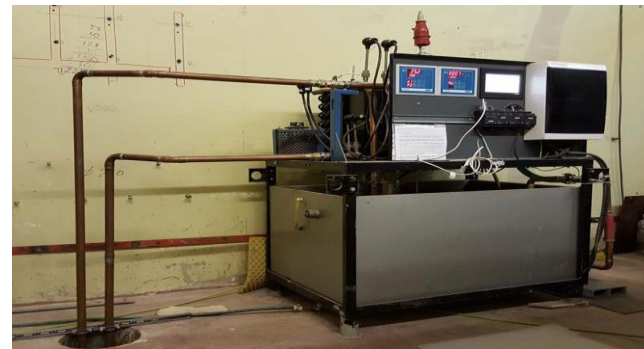
General view of the temperature control system
