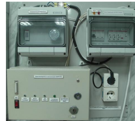
Interlocking and alarm system switchboard
