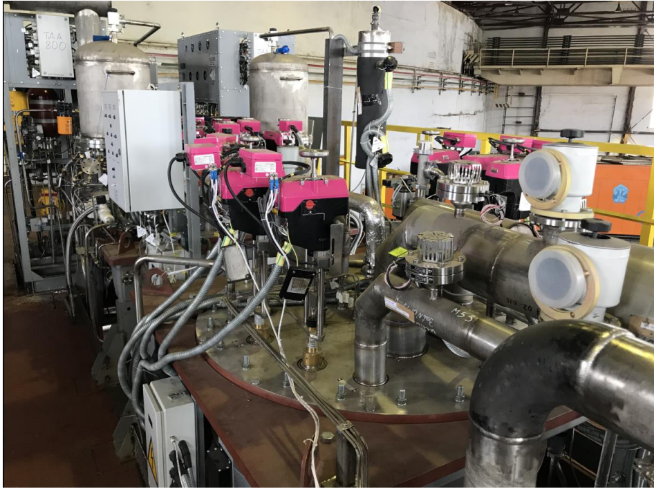
Fig. 3. Satellite refrigerator RSH-2000/4.5.
