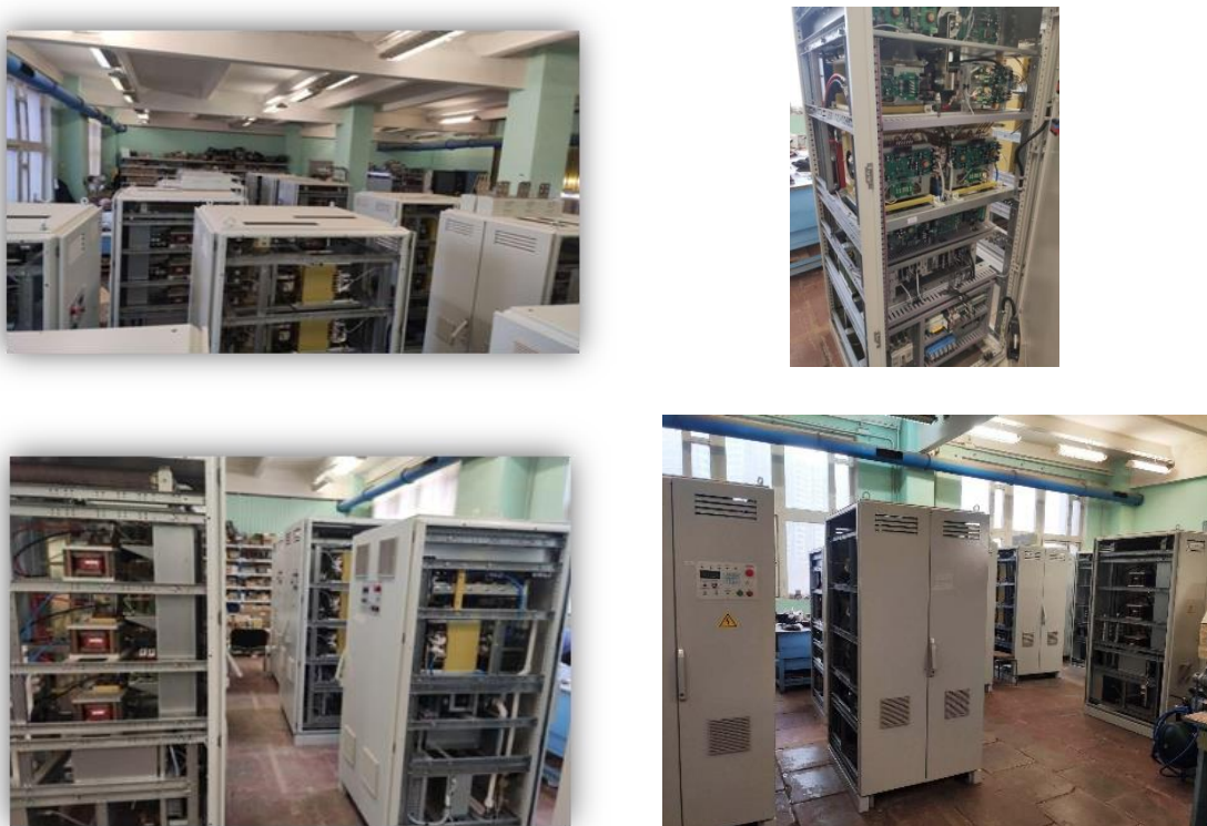
Fig. 15. PIT 11-50 power supplies
