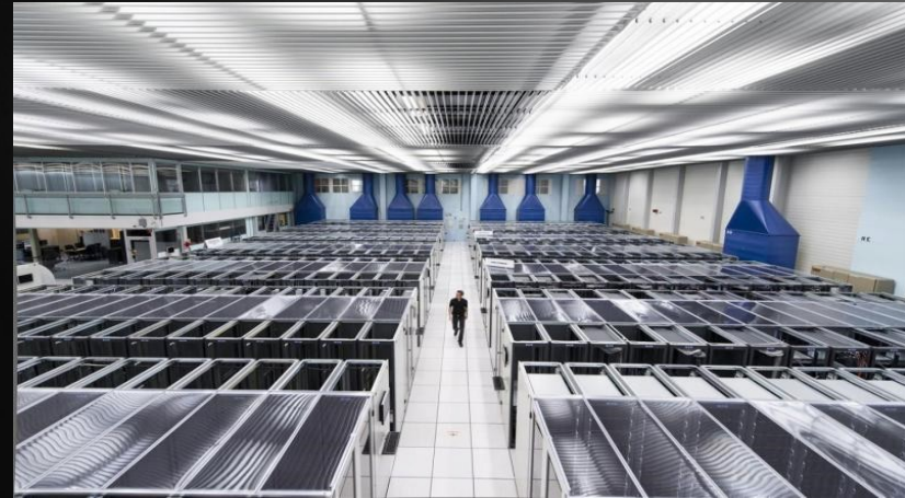
CERN data center
