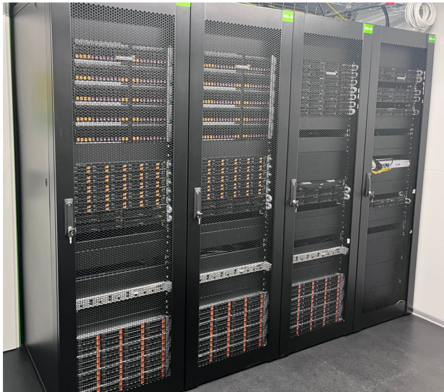
Figure 52: BM@N Modular Data Center server racks.
