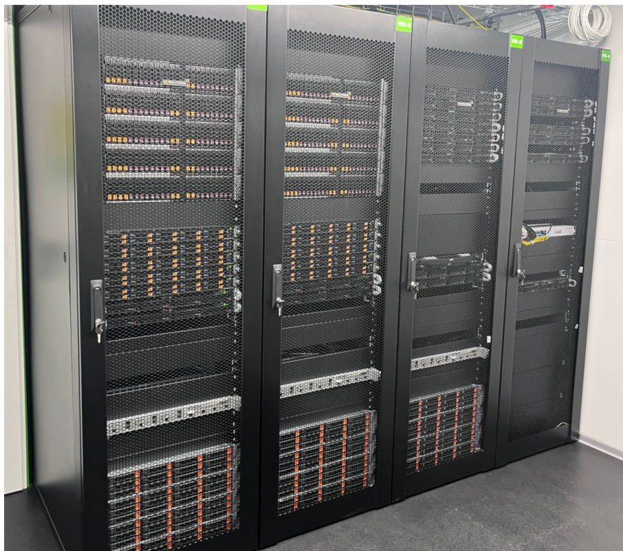
Figure 52: BM@N Modular Data Center server racks.
