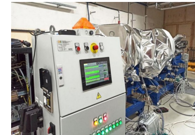
Two RF-stations are installed in the tunnel
