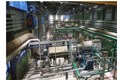
New compressor station will be commissioned in summer 2024
