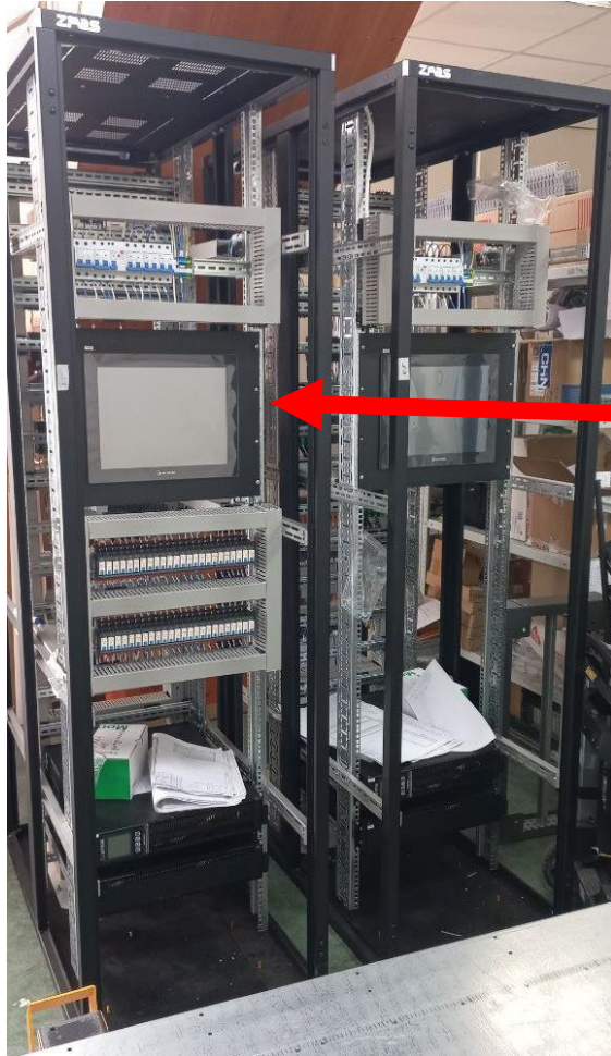
Distribution control rack
