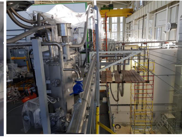
Strings for cryogenic pipes and cables hold
