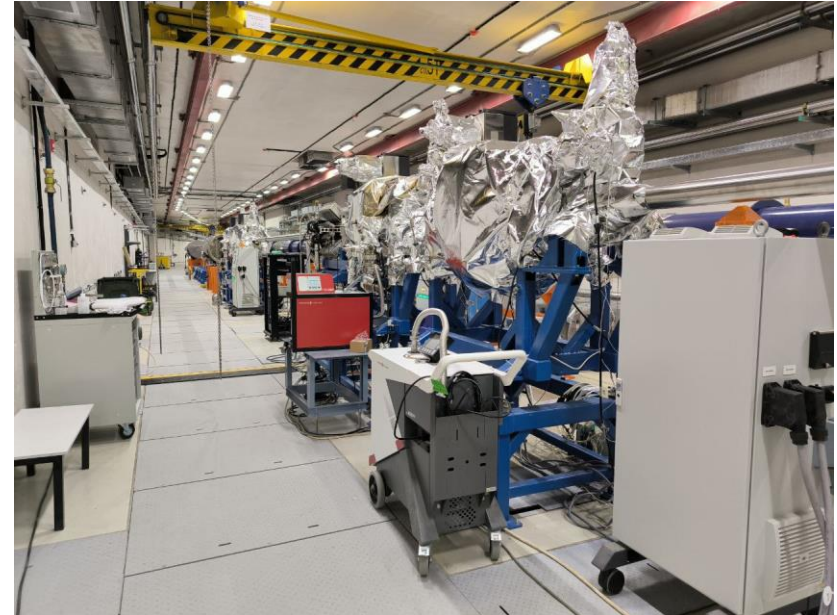
RF1 and RF2 in tunnel
