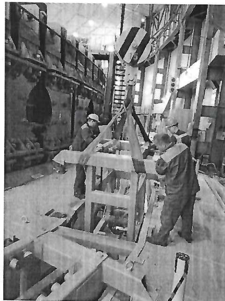
Fig. 1. Elements of the Booster-Nuclotron beam transport line during assembly.
