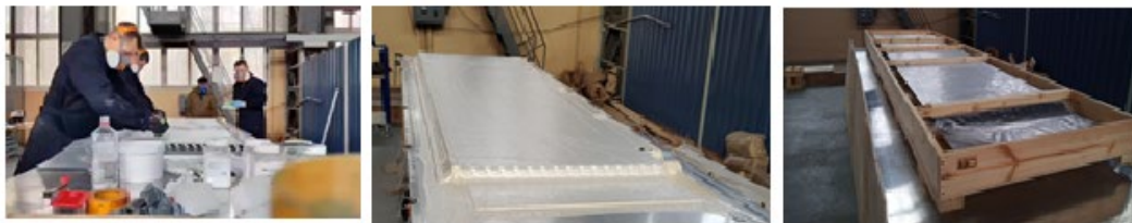
Fig. 54. Gluing process; module, under a vacuum pressure of 26 tons; finished module in a box
