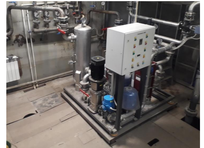
Independent water cooling module for RF generators
