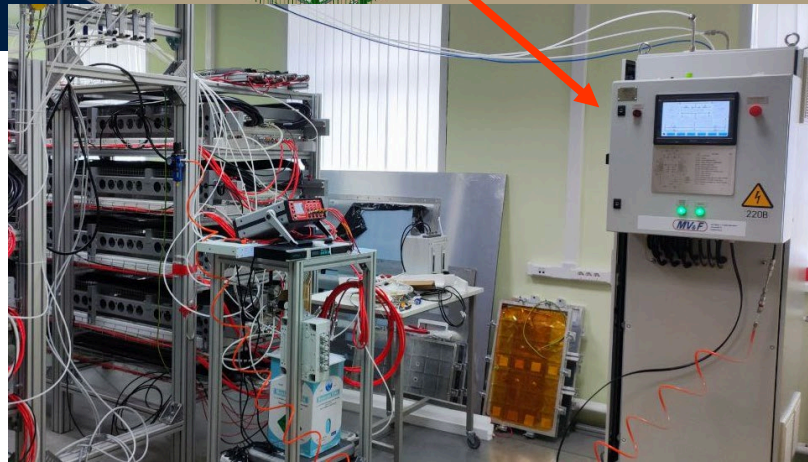
Gas mixture purifier (rack #4)
