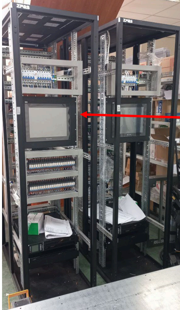
Distribution control rack
