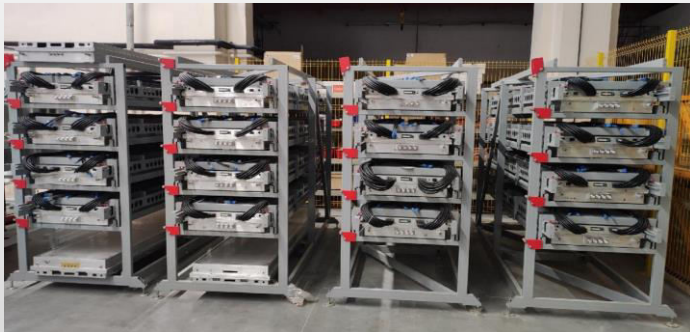
TOF modules in storage (28 in total)
