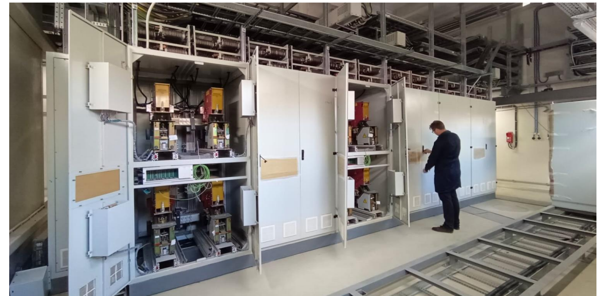
Energy evacuation system (including switches)
