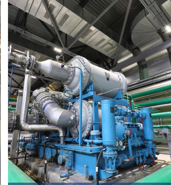
A new compressor (1 of 4)
