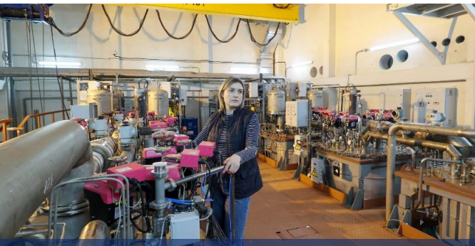
Cryogenic equipment in the collider building
