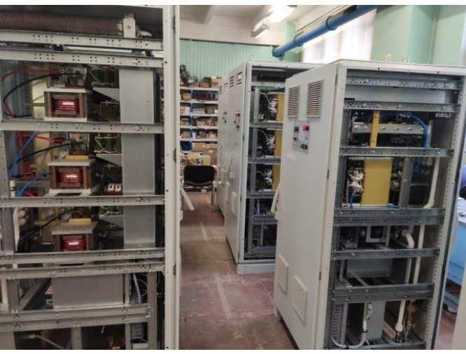
Power supplies are mounted at the collider. Completion – Dec'24
