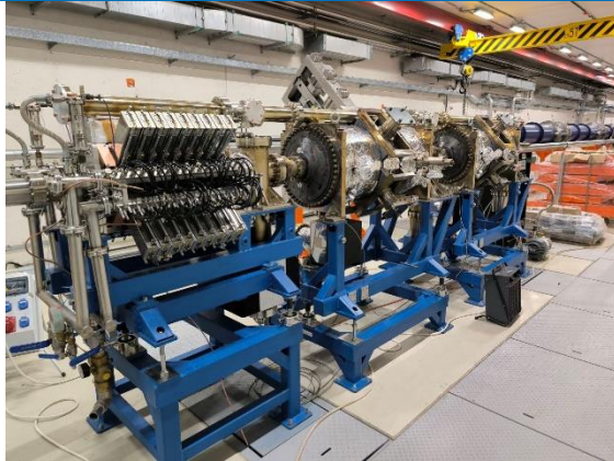
RF1 and RF2 in tunnel
