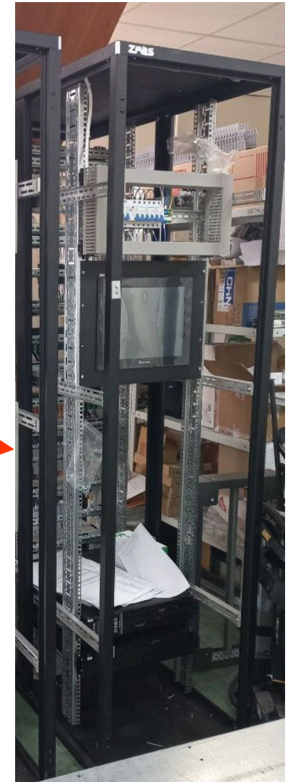
Automatic and control (rack #1)
