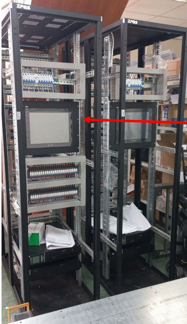
Distribution control rack
