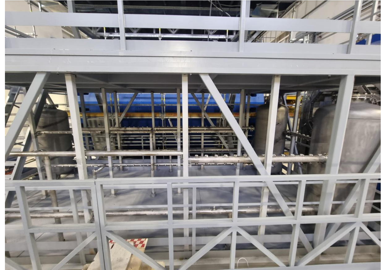
Water tanks & manifolds
