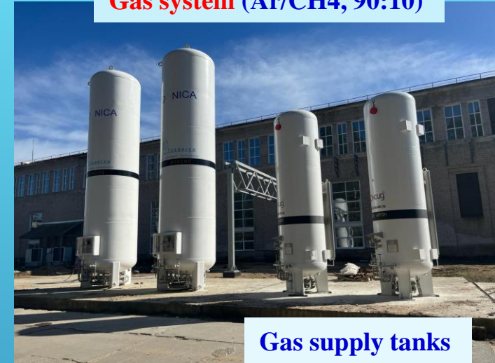
Gas system (Ar/CH 4 , 90:10)
