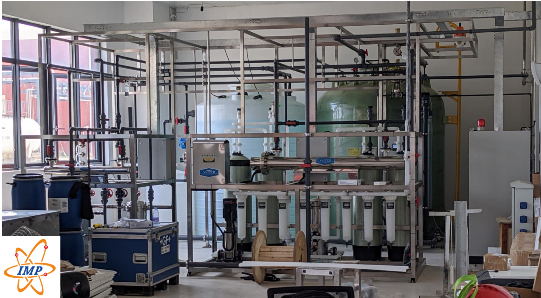
UPW plant at IMP
