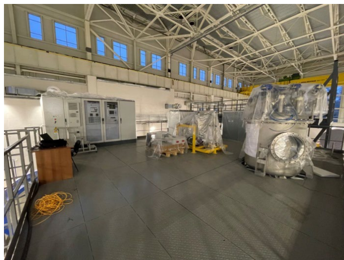
Figure 3. Placement of solenoid engineering systems on a cryogenic platform.
