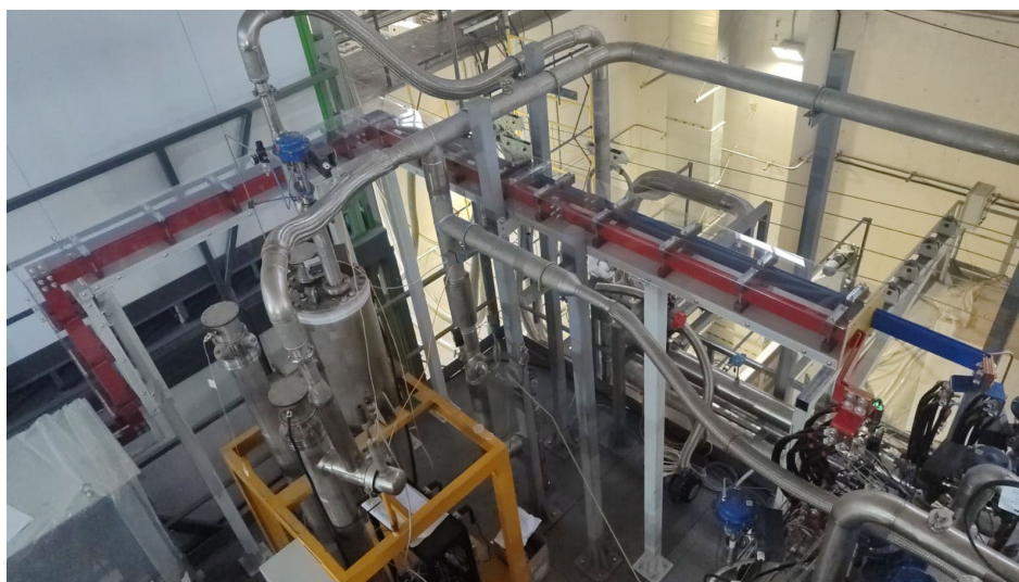
Figure 8. Busbar from the external resistor to the current leads of the SC magnet.
