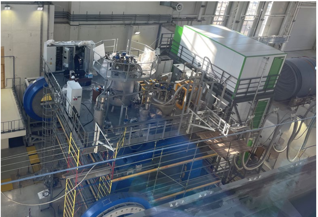
Figure 5. General view of the technological platform, with the installed equipment.
