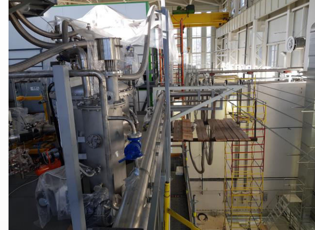
Strings for cryogenic pipes and cables hold
