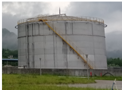
5000 m 3 LAB tank
