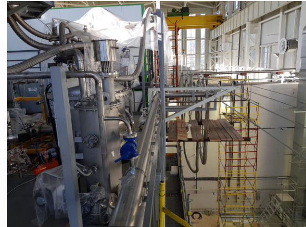
Strings for cryogenic pipes and cables hold
