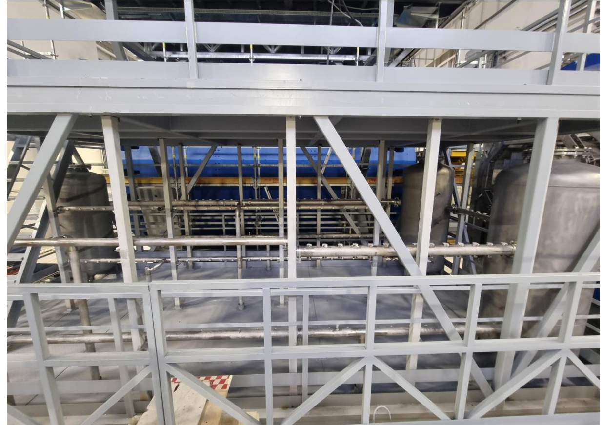
Water tanks & manifolds
