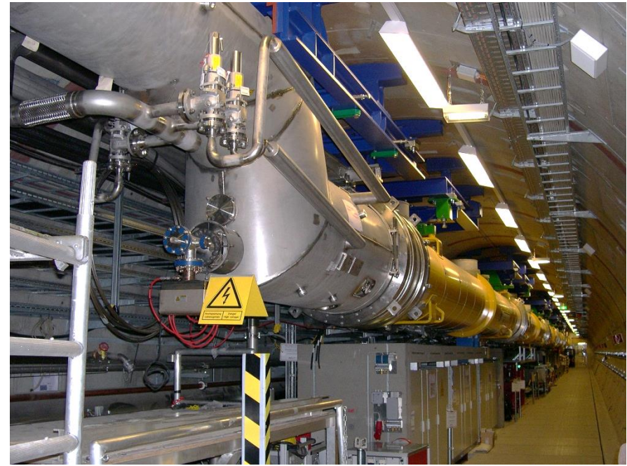
Assembled cryo-modules of XFEL, DESY, April 2015 (about 1000 of our T-sensors)
