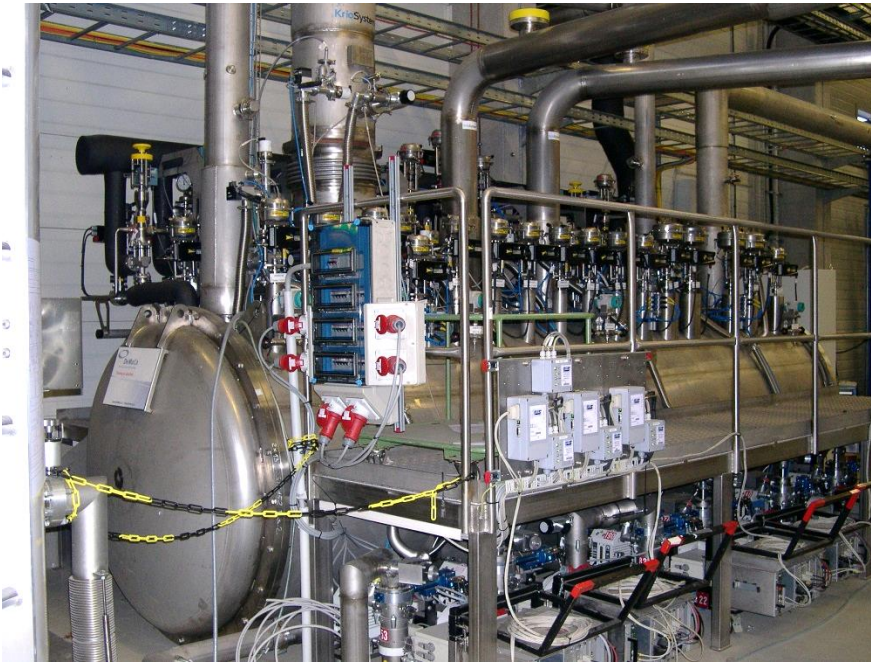
Assembled helium valve box at AMTF, DESY, December 2013
