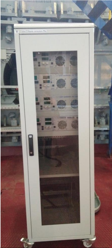
Control rack of correctors
